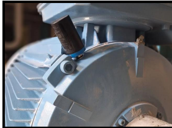
Contributor : Pascal ZAGAR (Regional Maintenance Manager CE)
